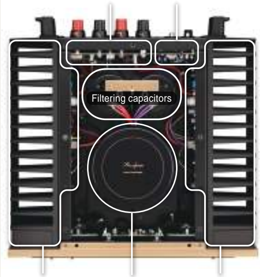
L ch power amplification section Toroidal transformer R ch power amplification section
